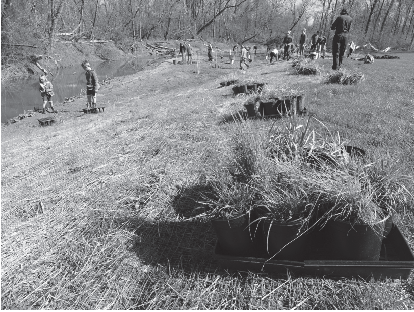
FIGURE 10. Floodplain restoration in process at Crystal Springs site located at the Leisure Creek Condominium Association. May 6, 2022. Photo by David P. Warners.
